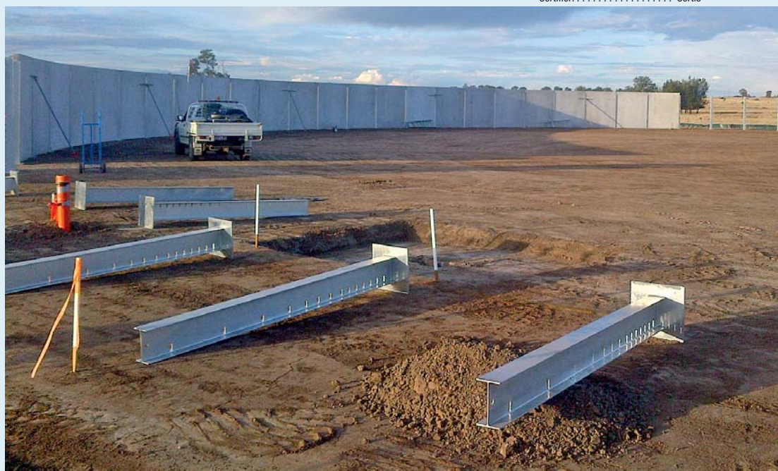
HUTCHIES is currently building a series of seven Water Gathering Stations (WGS) for Origin Energy in the Surat Basin. Shown is the first day's construction of a 12 megalitre Emergency Ballast Storage Tank (EBST) which is back up for the WGSs should the pumps fail. The EBST is 70 metres in diameter and has three-metre precast concrete walls with post tensioned steel cables running around the outside and finished with a poly liner.
