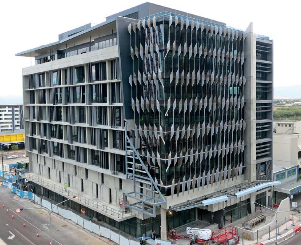
Removal of Hutchies' construction scaffolding has revealed a stunning new streetscape sculpture for Townsville at 420 Flinders Street.
