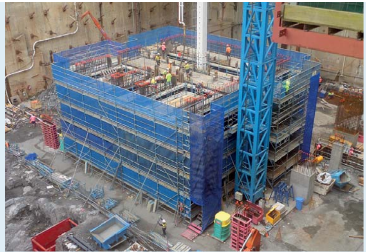
WORK is continuing well on the carpark project at 111 Mary and 222 Margaret Streets in Brisbane since Hutchies took over the site in mid-March this year.
